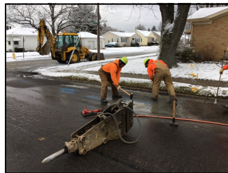
A Distribution Department crew working on a water main break at West 35th Street and Washington Avenue.
