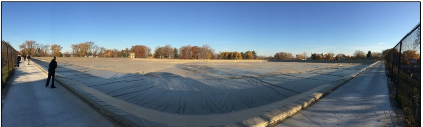
A panoramic view of the new Sigsbee Reservoir floating cover after project completion.
